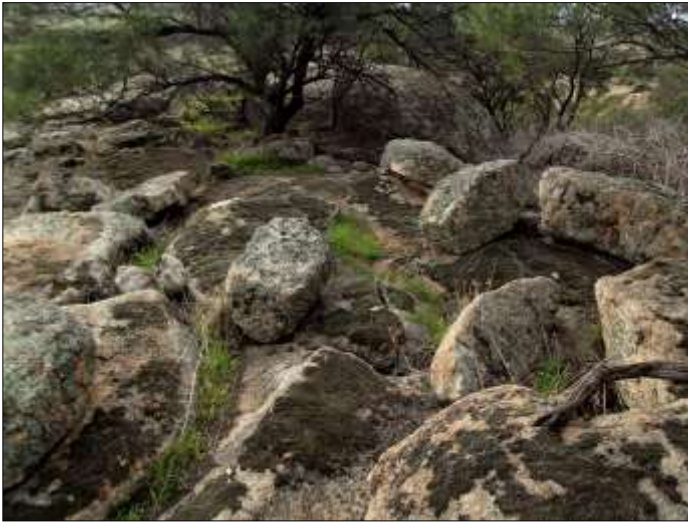
The remains of a collapsed structure, west side of Pyramid Hill. Photo copyright © Rex Gilroy 2018.
